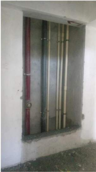
Water supply pipework within the ducts
